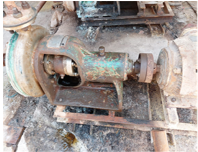
Fig. 3. Sulfuric acid pump
