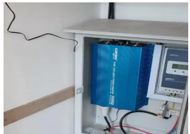
Fig. 5: Converter and controller charger of the studied system.
