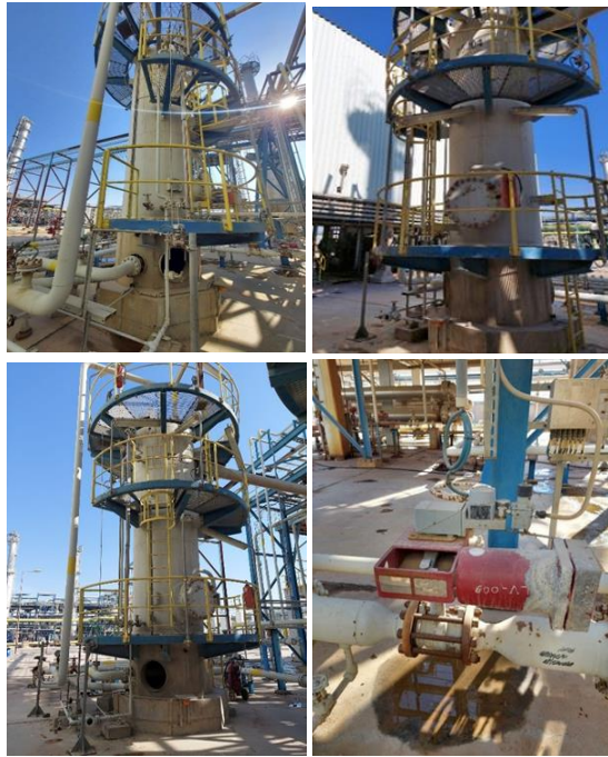
Fig. 3: D5204 in Basrah Refinery.
